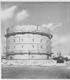
NEARLY COMPLETED is the installation of a 20,300-barrel storage tank. Going up, rear, is the 23,300-barrel tank. E INSTALACION di un tanki di 20,300-barrel ta casi cila. Banda patras, un tanki di 23,300-barrel ta bai laria.
